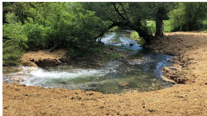
Recently installed rock weir with plunge pool creating cover for Tainter Creek brown trout. Streambanks have been mulched and seeded. / Photo credit: Wisconsin DNR
