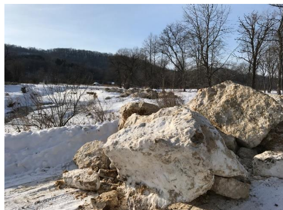
Rock staged along Weister Creek ready to be installed. / Photo credit: Wisconsin DNR
