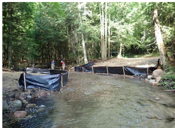
Red River project site where the culvert was removed and replaced with instream crossing. Silt fence to retain runoff until slopes are stabilized. / Photo credit: Wisconsin DNR
