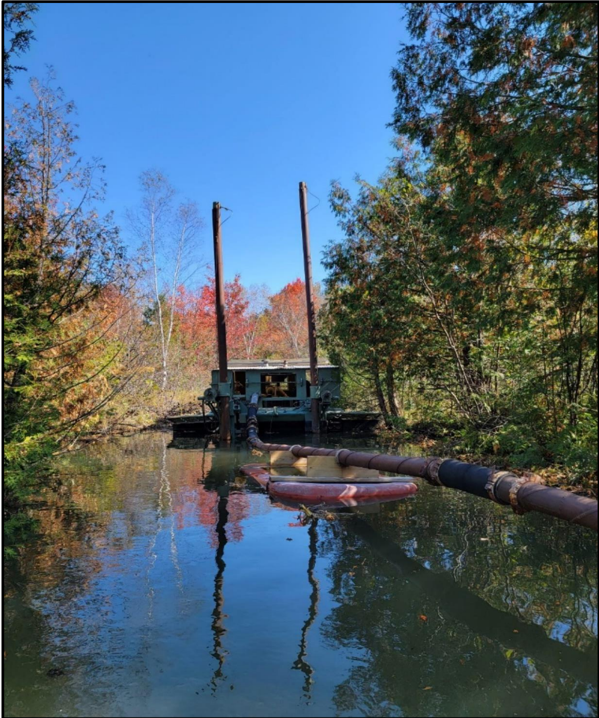
Dredging at the confluence of the Stillhouse spring pond and Lost Spring spring pond outlet creeks / Photo credit: Wisconsin DNR
