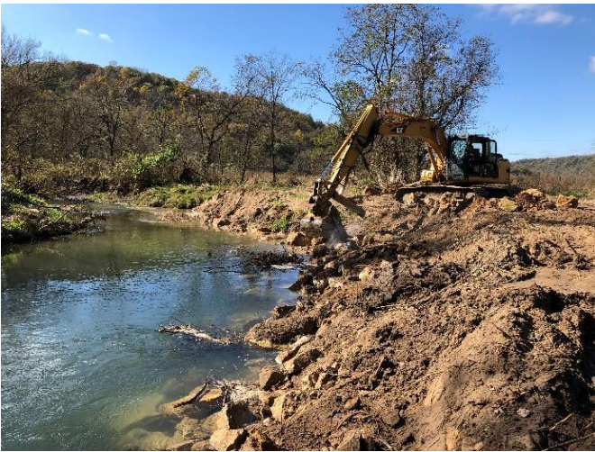
Rush Creek streambank being stabilized with logs and root wads incorporated into the rock. / Photo credit: Wisconsin DNR
