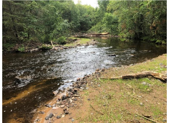
Point bar shortly after construction on the Hunting River. / Photo credit: Wisconsin DNR
