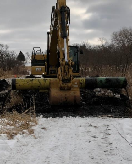
Removal of failing tin whistle on Tichigan Creek. / Photo credit: Wisconsin DNR
