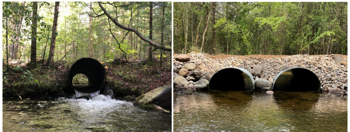
Culvert before replacement (left photo) and after replacement (right photo). / Photo credit: Wisconsin DNR
