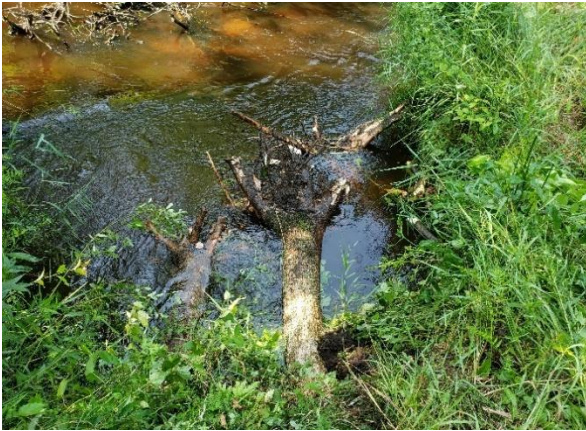
Root wad structures installed on sill installed on Little Roche-A-Cri Creek. / Photo credit: Wisconsin DNR
