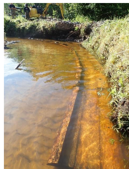
Installation of jetted bank cover on Fordham Creek. / Photo credit: Wisconsin DNR
