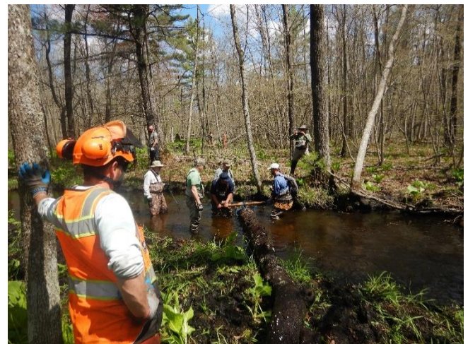
Wild Rose crew and partners moving a log for installation of a trout habitat structure. / Photo credit: Wisconsin DNR
