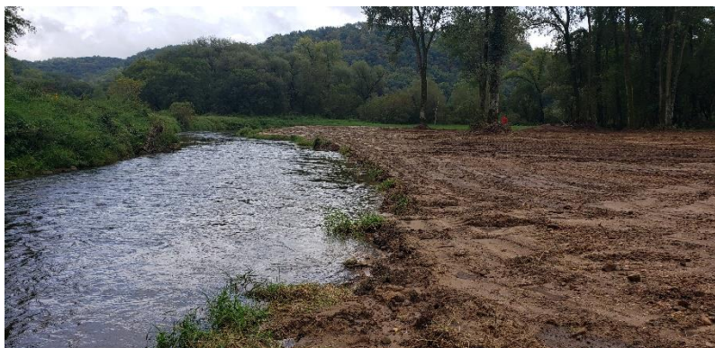
Streambank sloped to connect river to floodplain on the West Fork of the Kickapoo River. / Photo credit: Wisconsin DNR
