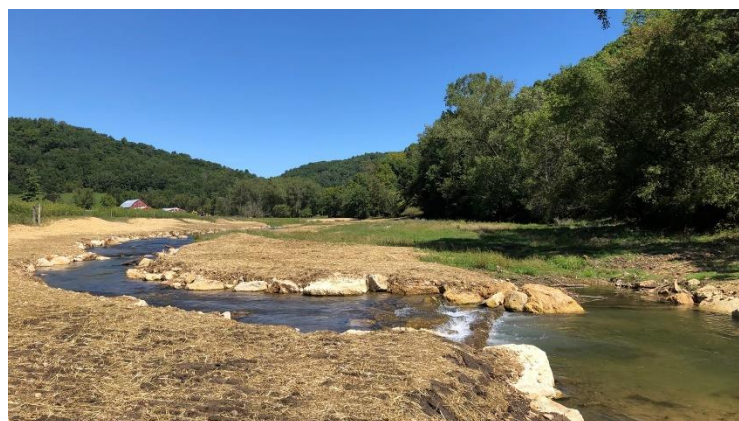
Coon Creek rock weir with cross channel log incorporated at the bottom and a small / Photo credit: Wisconsin DNR
