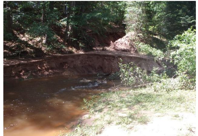
Eroding hillside and streambank on South Fork of the White River. / Photo credit: Wisconsin DNR
